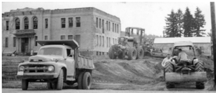
The brick school stood from 1910 to 1966, razed to make way for medical clinic.
